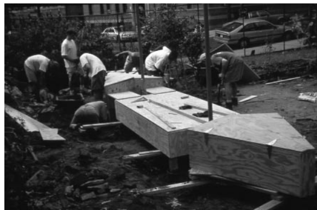
Children building alongside adults. Much of the work involved in building a children’s area does not require a skilled crafts person and can involve both parents and children.
